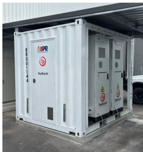
RedEarth's containerised Dingo solution
