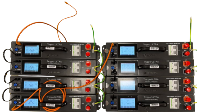
This is a completely wired battery pack.
