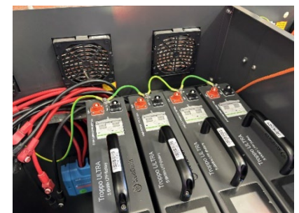
Daisy chain the earth cables (4 battery example)
