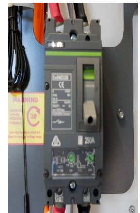
Battery System D.C. Isolator
