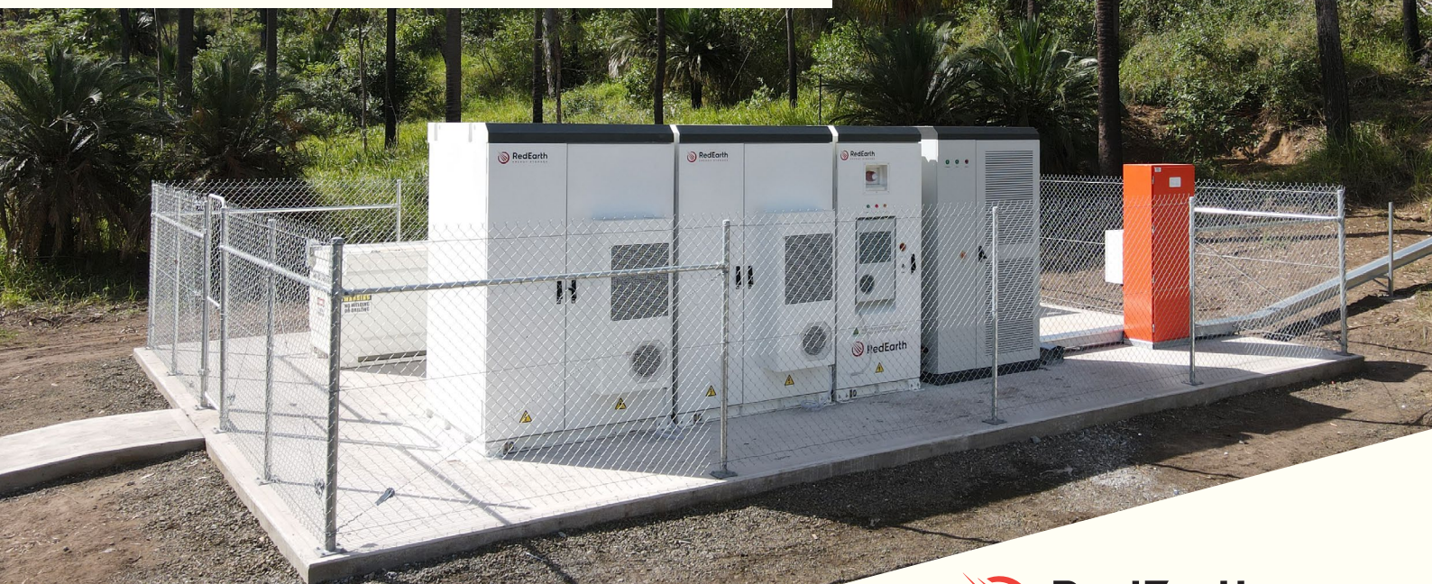
Pictured: An off-grid RedEarth commercial system in a caravan park in Carnarvon Gorge, QLD.
