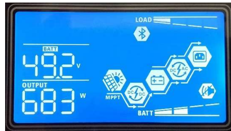
Day Time – Solar power helping the battery to power the loads
