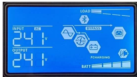
Night Time – Generator powering the loads and charging battery
