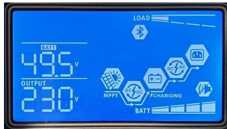
Day Time – Solar power charging battery and powering the loads
